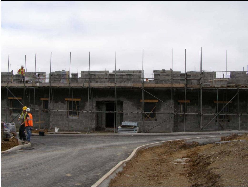
Local Needs Affordable Housing – part of the 9 units currently under construction at Exford (© ENPA)
