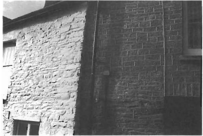
The pleasant lime-washed stonework to the left hand side contrasts sharply with the poorly pointed wall to the right ... a form of stonework pointing that is not encouraged.
