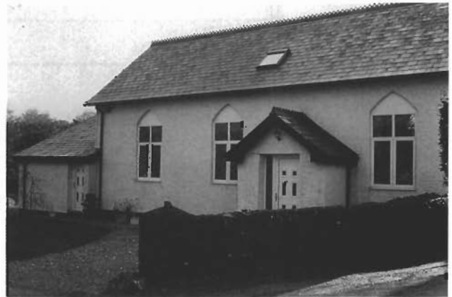
Originally a chapel, this building has suffered at the hands of over-enthusiastic restorers. The windows and rooflight, and more particularly the UPVC doors, are totally unsuitable and probably replaced fine timber versions that should, if possible, have been repaired and retained.
