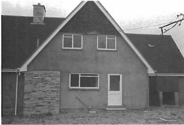
The ad hoc use of different materials does little to improve the appearance of this building.
