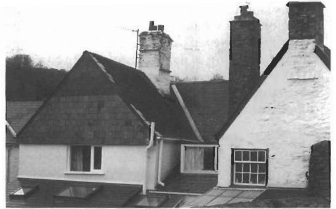
These new windows do little to improve the appearance of this older building, and being at the back is no excuse!
