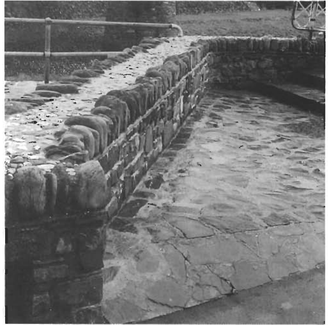
Changes in levels, however slight, can be a hazard to people with disabilities.
