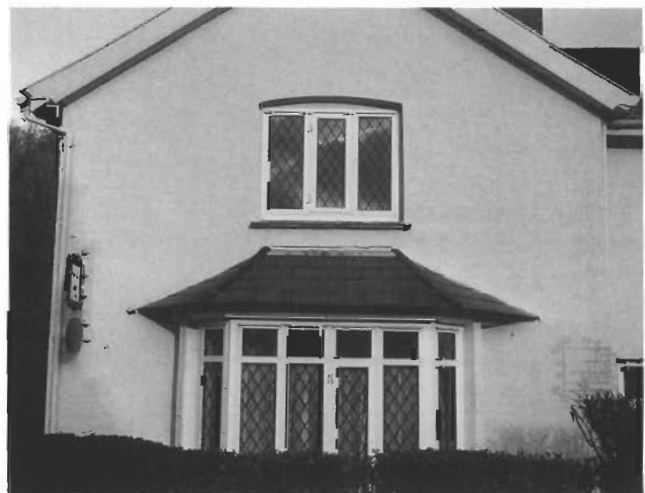
Replacement UPVC windows — the example shown here even has applied leaded lights — are inappropriate in older buildings.
