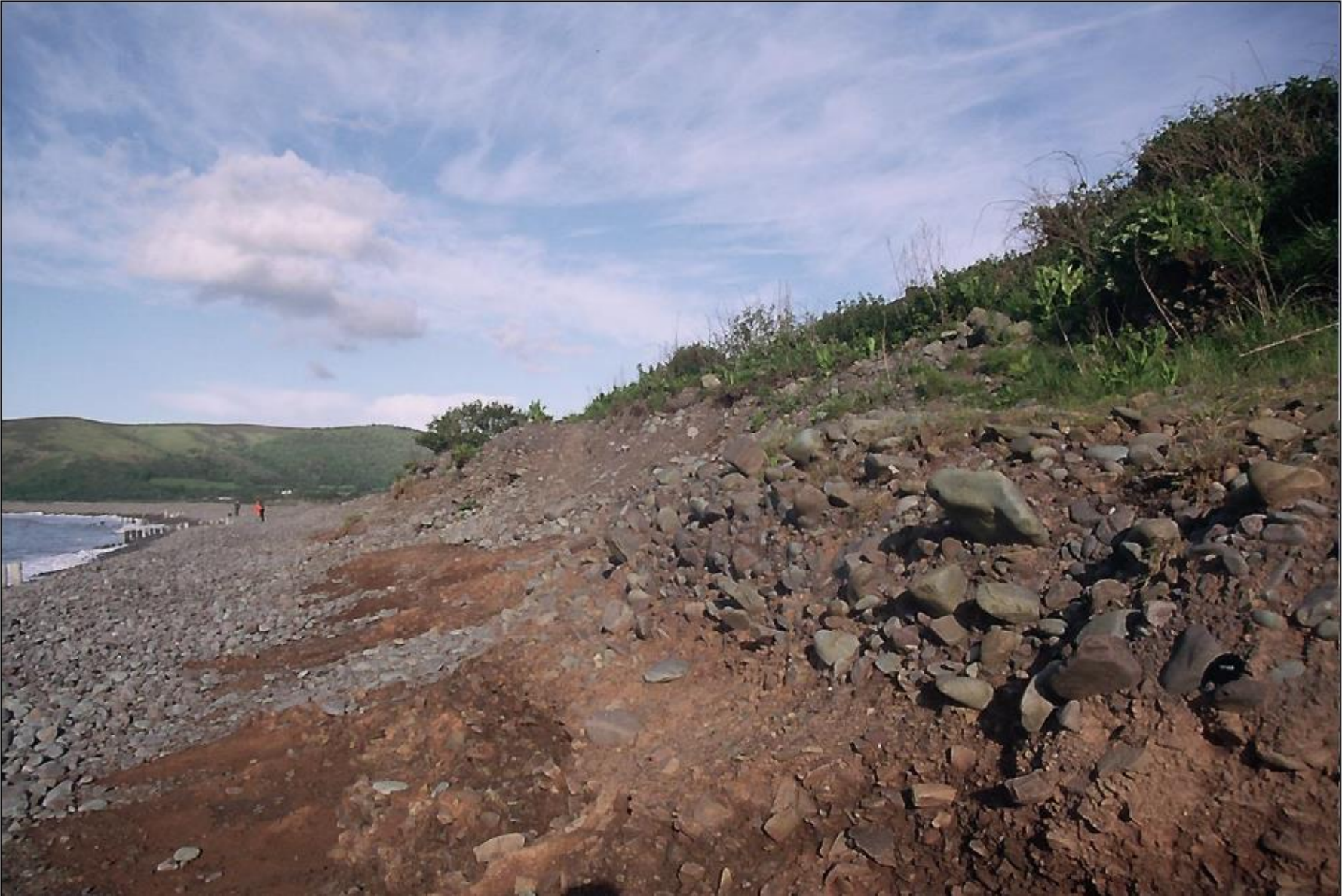
Resource 5 - Erosion at Porlockford Cliff
