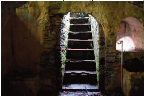
Fig. 8 Interior north wall, showing stair and doorway, extant niche (right) and remains of blocked niche (left); (photo ref: SRB 9745).
