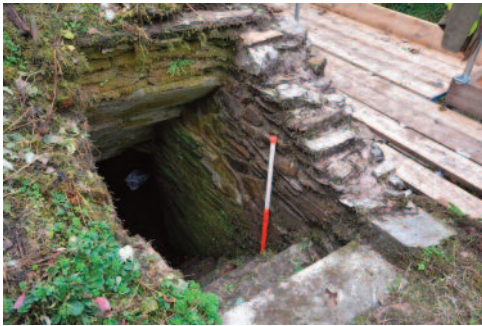
Fig. 6 West wall of stair, looking south-west, showing original masonry below, repair above (photo ref: SRB 9742).
