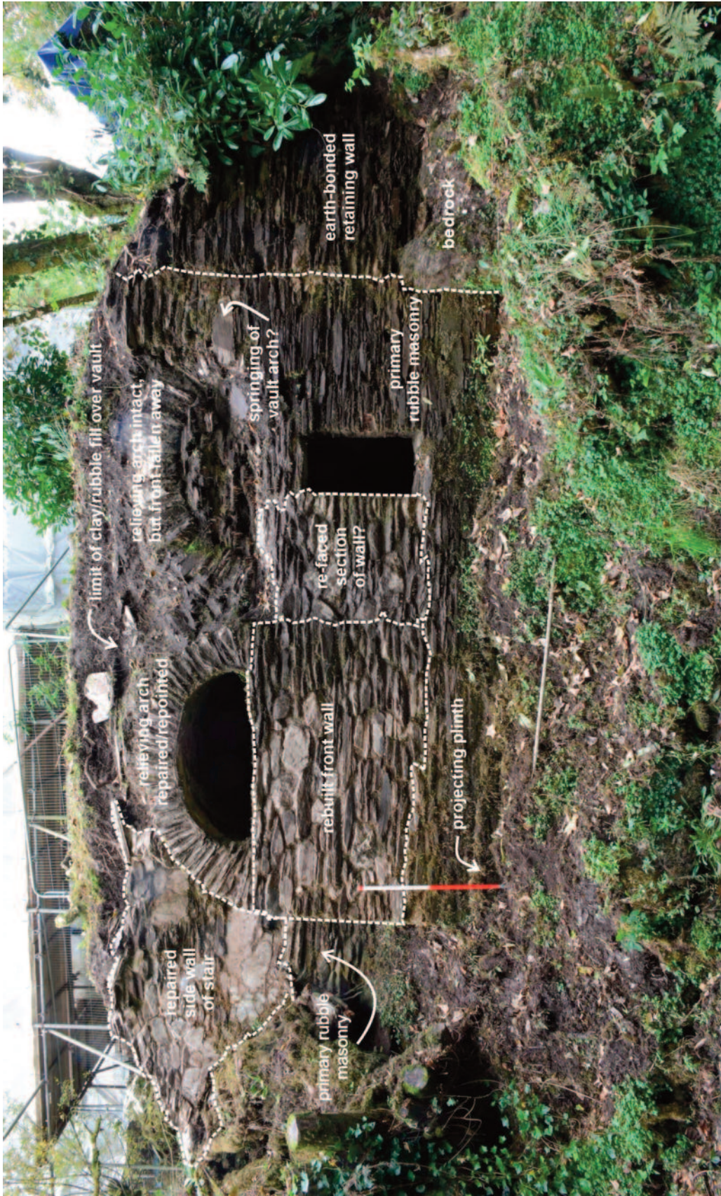
Fig. 5 West elevation annotated with the lines of masonry breaks and other details (photo ref: SRB 0037, cropped).
