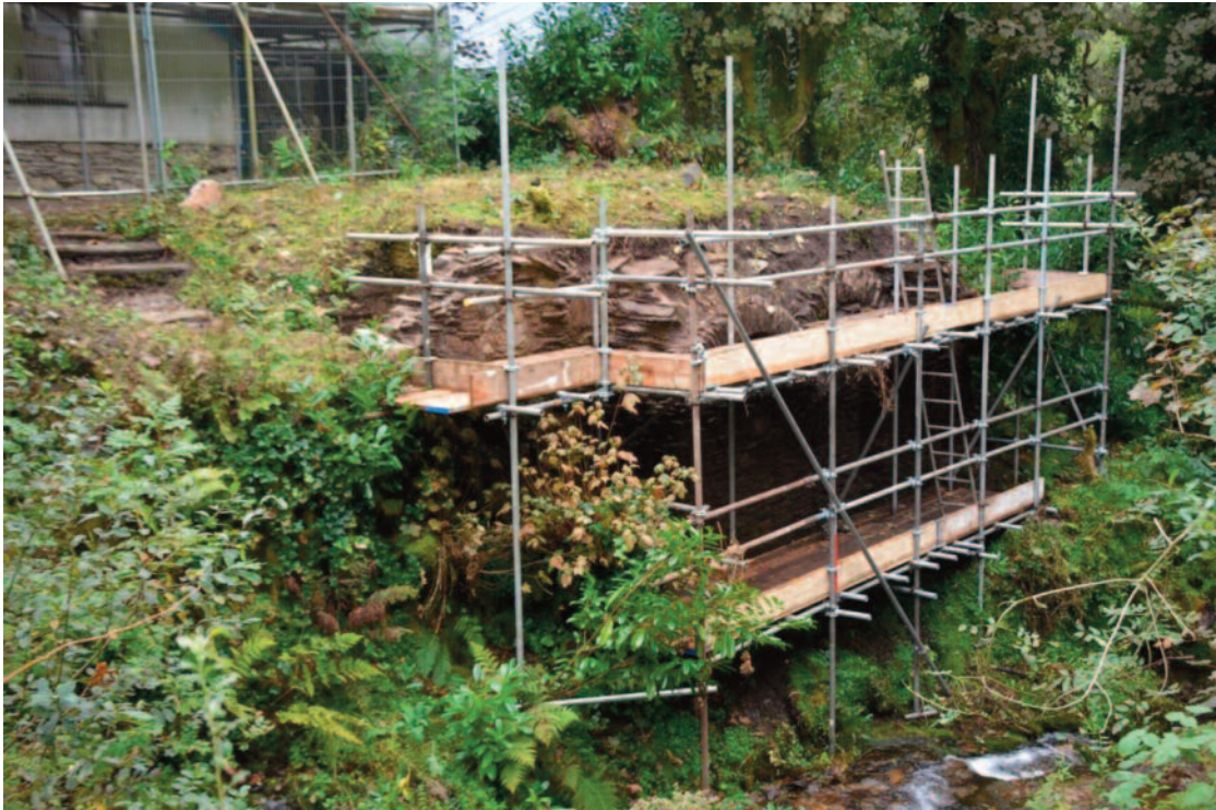
Fig. 4 The building from the north-west, with scaffolding in place, 28.ix.16 (photo ref: SRB 9696).
