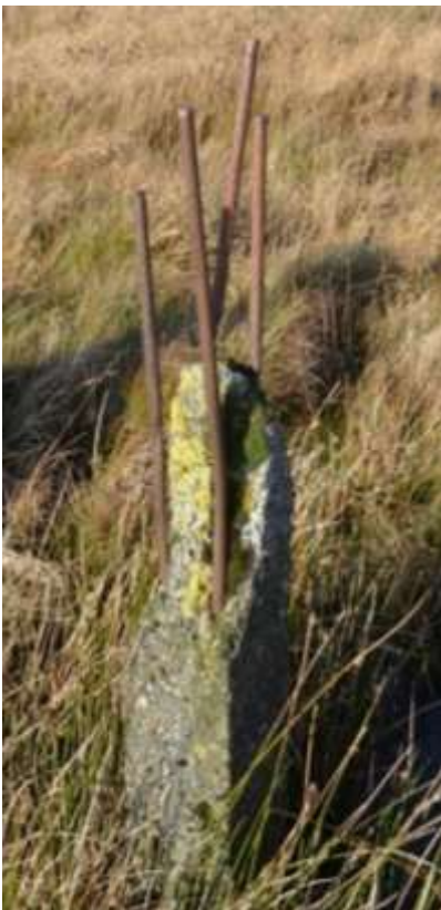
Figure 88: Deteriorating concrete post
