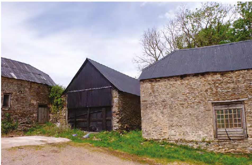
Fig 46 North end of yard with LB7 to left, wagon shed (LB8) middle, and barn (LB9) to right.
